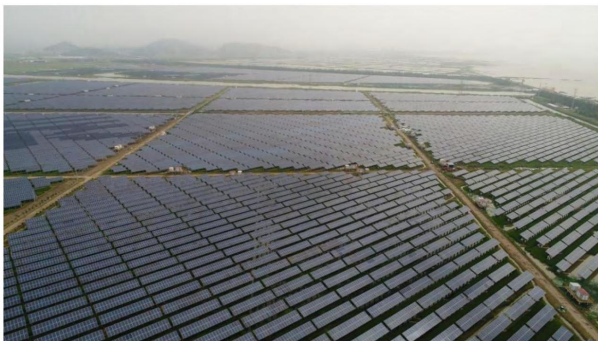
Figure 2 Photovoltaic power generation area
