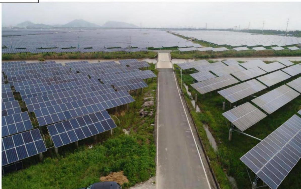
Figure 1 Photovoltaic power generation area
