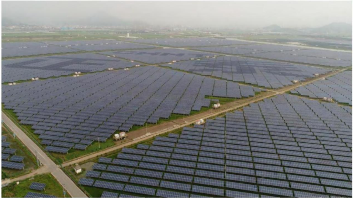
Figure 3 Photovoltaic power generation area
